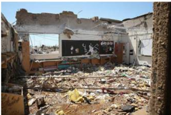
Classroom at Plaza Towers Elementary School
